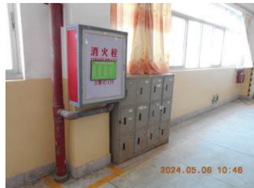
Fire extinguishers and Fire hydrant.JPG
