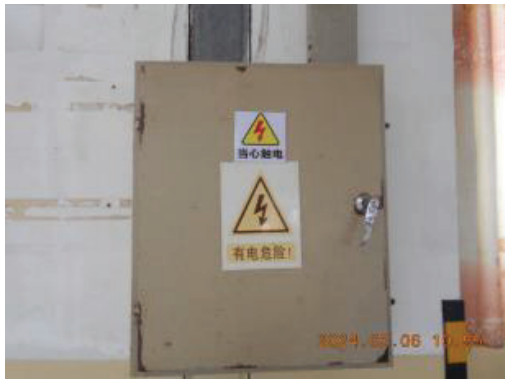
Electrical wiring box with warning sign.JPG
