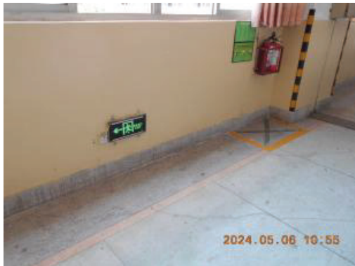
Aisle with the evacuation sign.JPG
