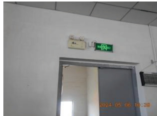
Exit sign and emergency light.JPG
