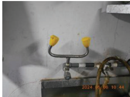
Eye washing facility.JPG
