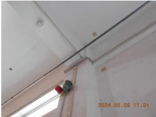
Fire alarm and smoke detector.JPG
