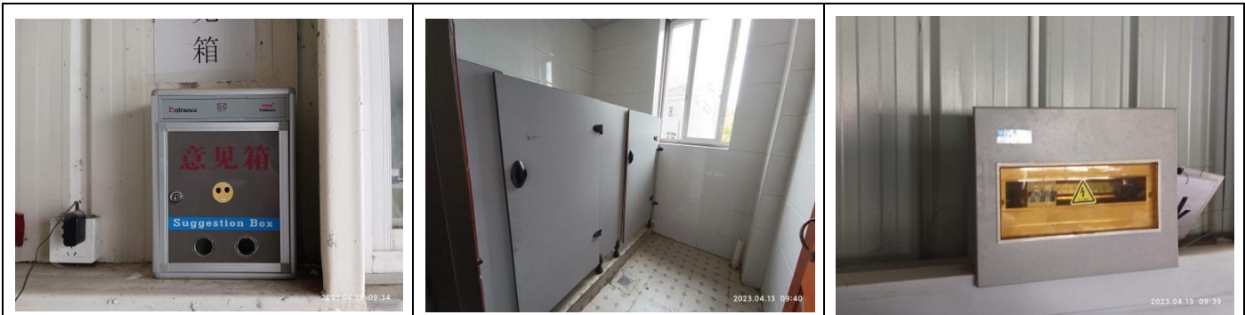
Suggestion box Clean toilet Electrical control panel
